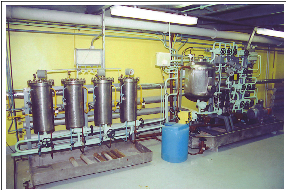
Figure 2.1.4-6. Selective sorption and reverse osmosis liquid waste treatment facilities at Zvezdochka shipyard.
