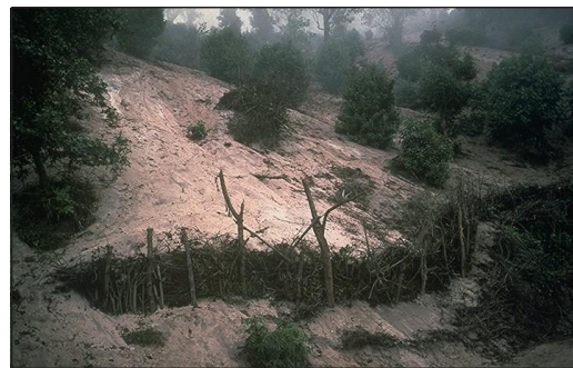
Picture 2 Application of barriers for the prevention of erosion of the terrain caused by construction works
