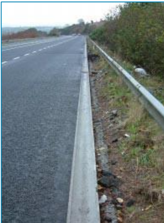
Picture 8 Drainage system composed of gutters
