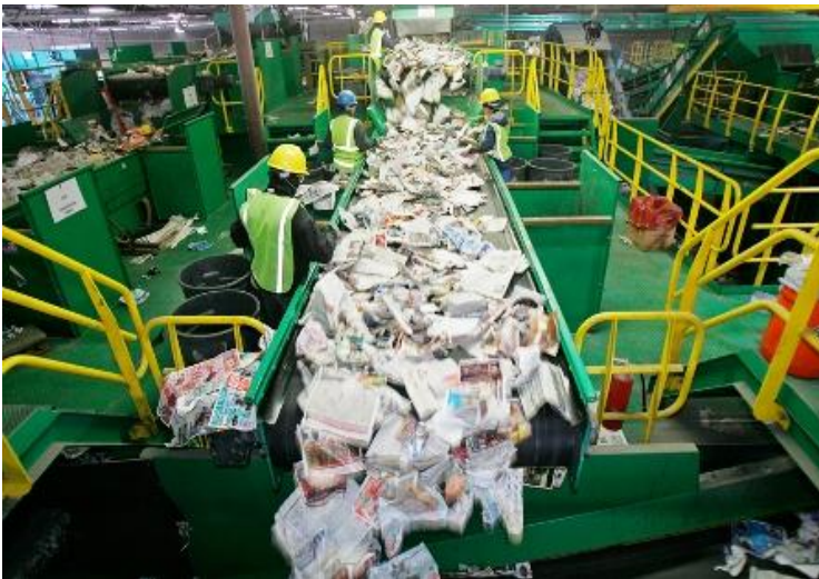
Figures 3, 4. Waste sorting facility examples
