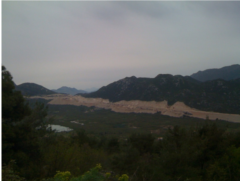
Photo 7: Southern Section: Ploče Interchange – BiH border. Looking southwest, toward Ploče Interchange from existing highway along section of A1 under construction.
