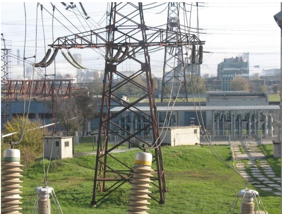
Figure 5. The switching port of pressure conduits
