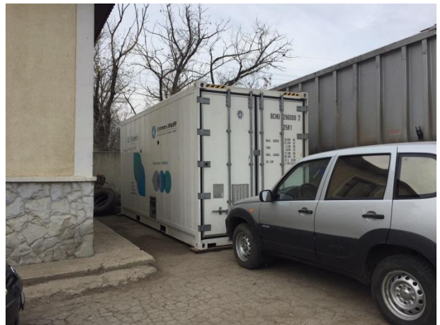
Photo 10: Leachate treatment plant delivered (Ciocana)
