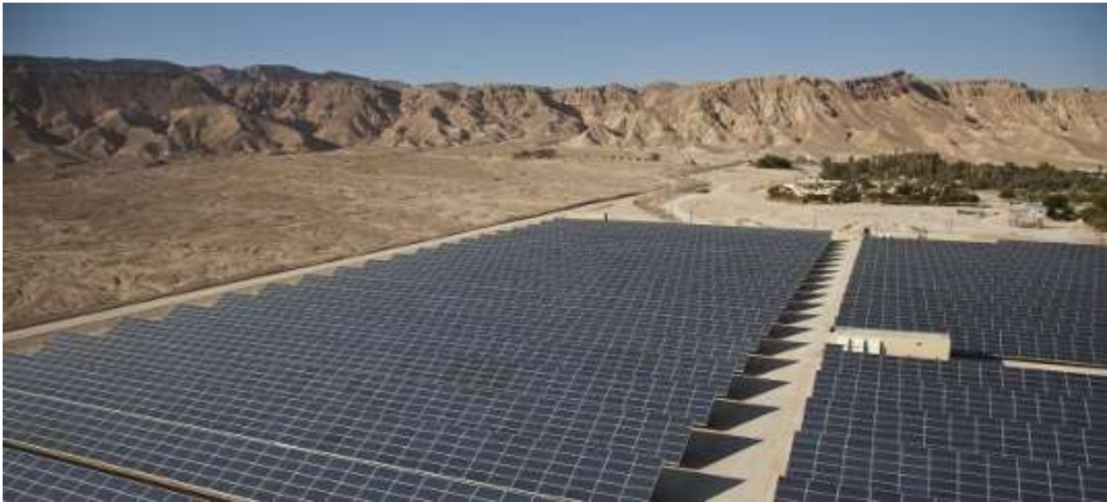
Figure 3: Typical PV Power Arrays Composed of PV Panels
