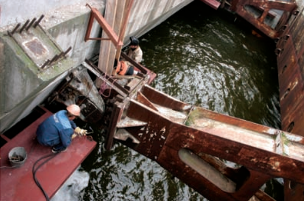
Construction of a flood protection barrier for St Petersburg is nearing completion thanks to funding from the Northern Dimension Environmental Partnership, which is supported by nine donors.
