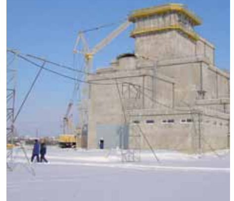
ISF-2 Processing Building
