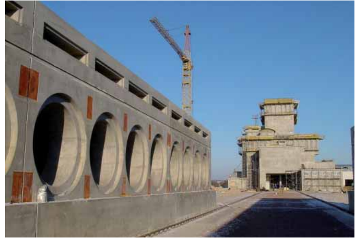
Concrete spent fuel storage modules
